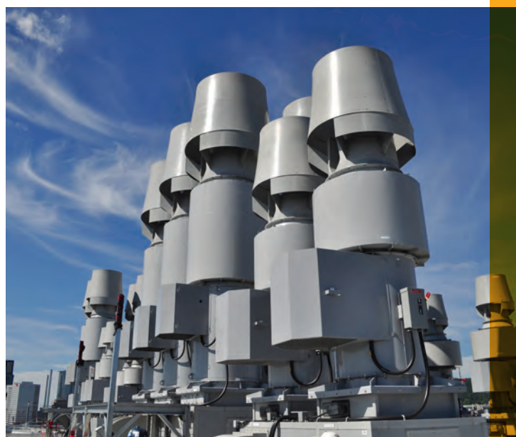
Axijet-V 4450 Coated Steel High Plume Fans (University of Montreal Teaching Hospital)
