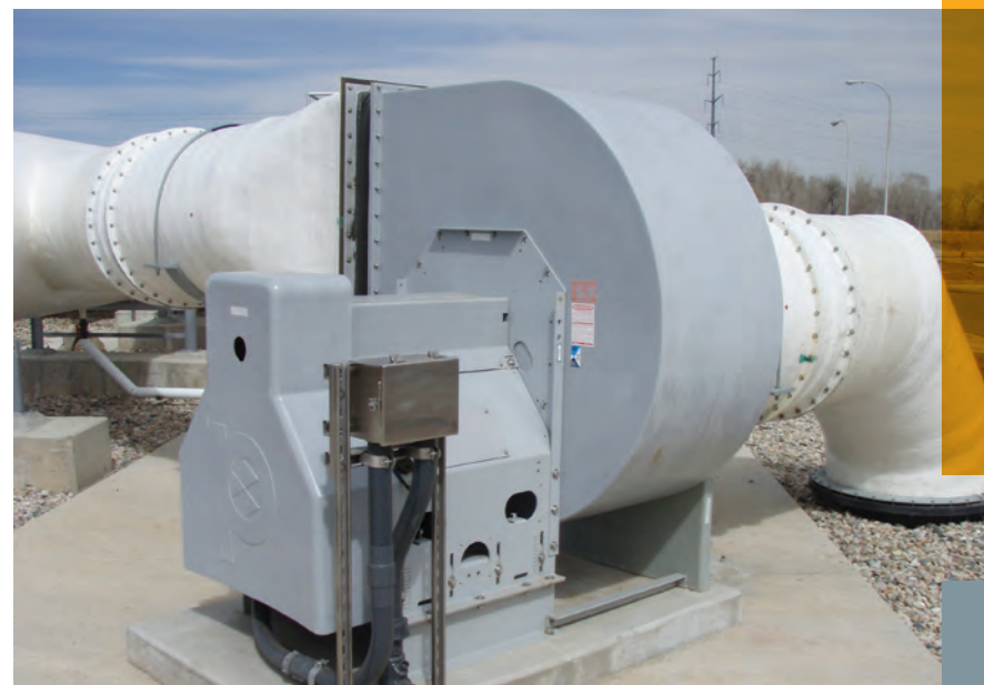
DHK 3650 Fiberglass Fan (City of Fort Collins Water Reclamation Facility)
