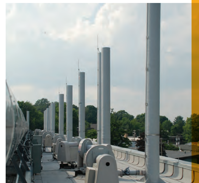
Perchloric Acid MVT Fiberglass Exhaust Fans (Columbia University Geochemistry Laboratory)
