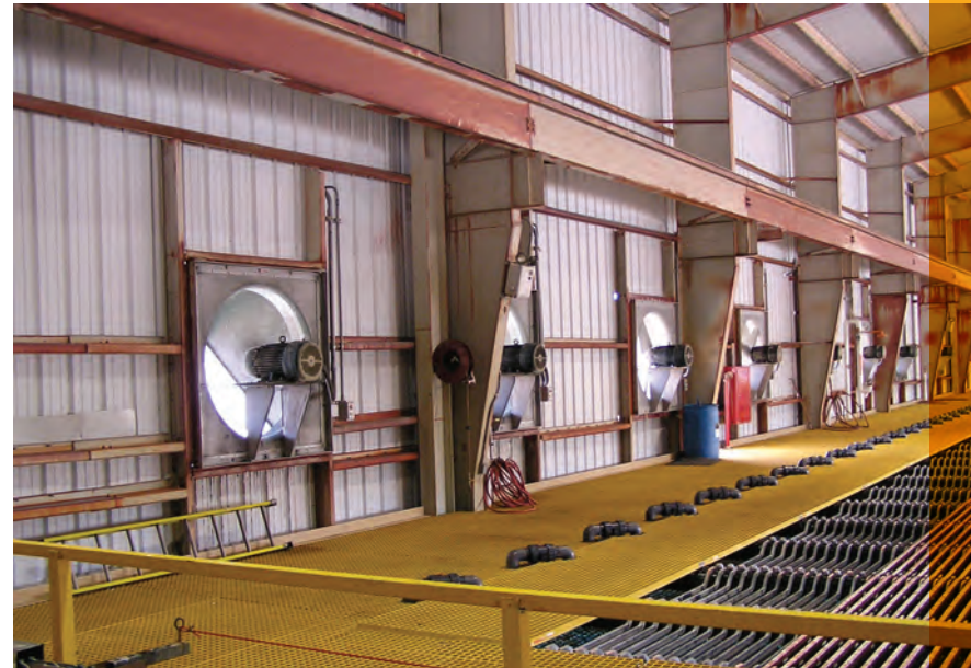
AXPR 54 Fiberglass Wall Panel Fans (Carlota Copper Mine Processing Plant)
